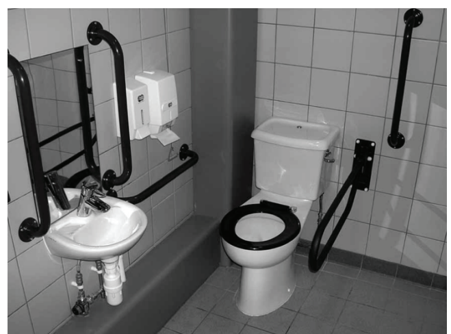
Figure 3: The unisex accessible cubicle (note: alarm incorrectly installed) (Bichard et al., 2006)
